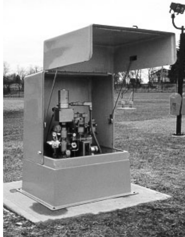
Figure 4.0 Below Ground Regulator with Fiberglass Cabinet.
